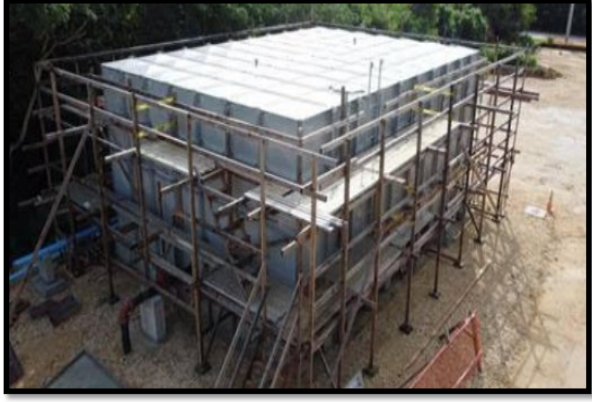
Dandan Temporary Water Tank
